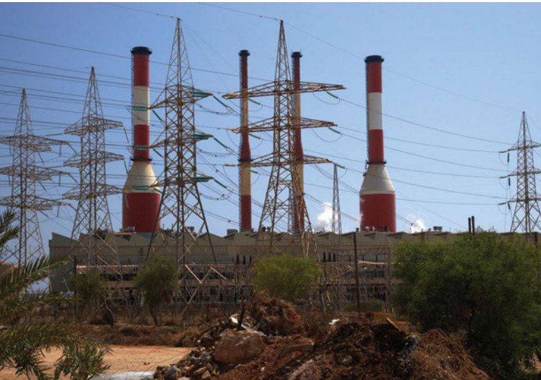
Oil-fired power station in Cyprus – indirect costs are a very high proportion of total costs in electricity generation
