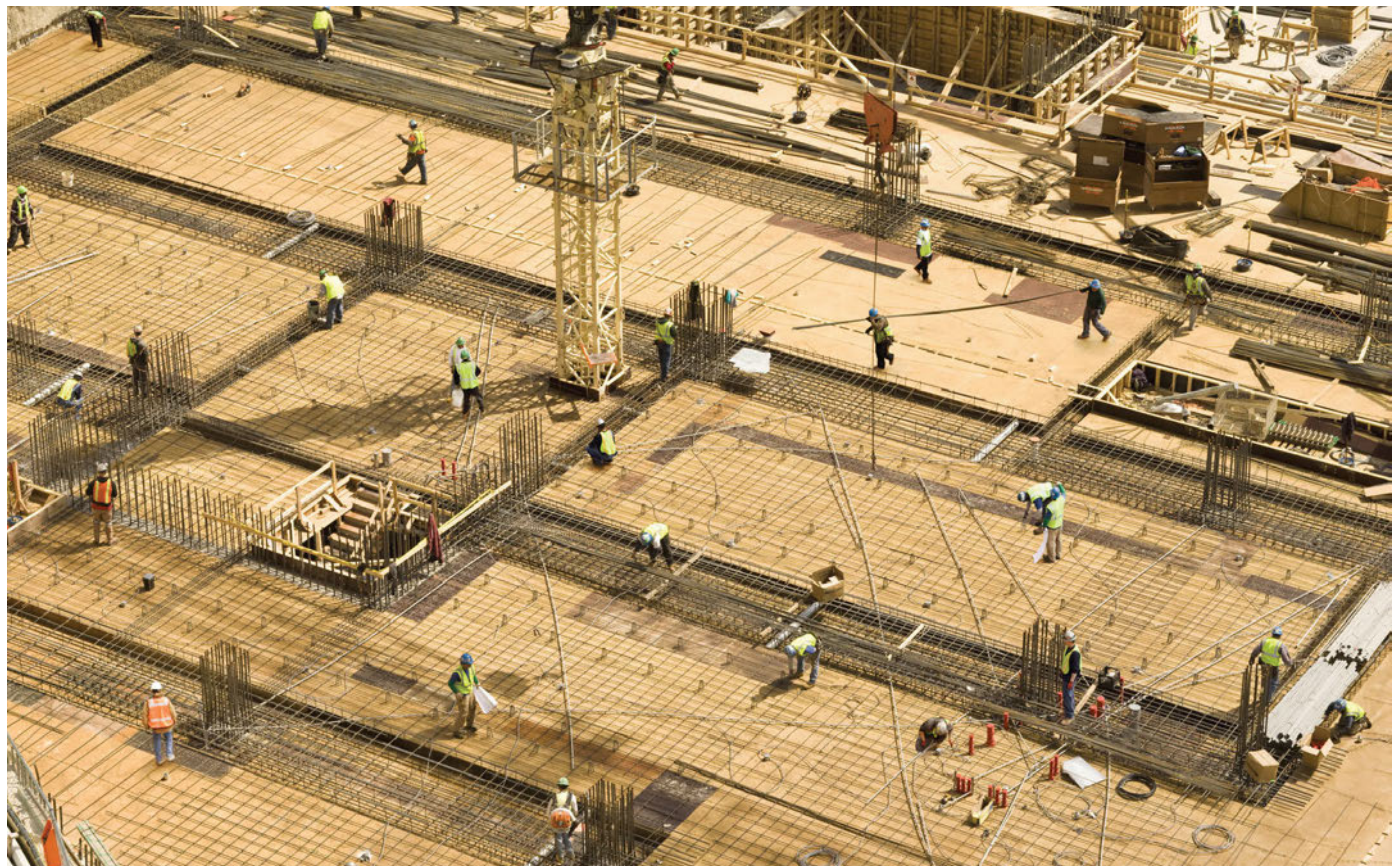
This construction site in the USA should follow all health and safety laws to protect its workers
